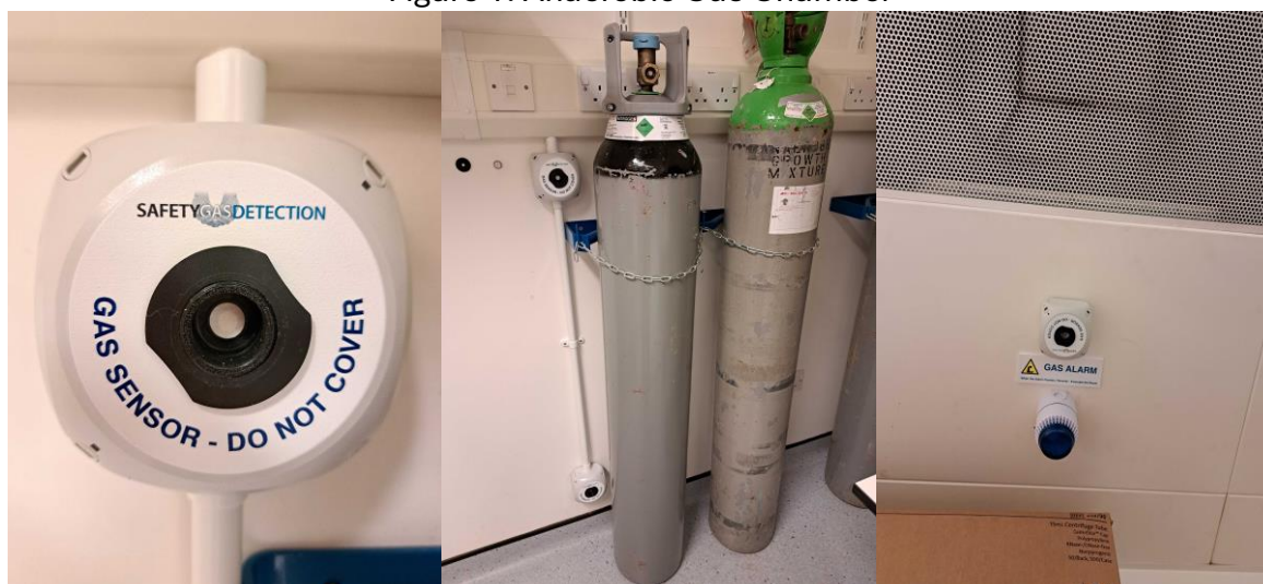
Figure 2. Gas sensors placed by the gas cylinders in A.4044 to detect any gas leaks
