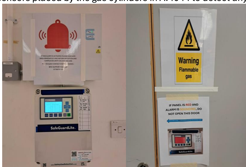
Figure 3. SafeGuardLite gas monitoring system. If the panel turns red and alarms do not enter the room. Alert the required personnel as shown on the sign.
